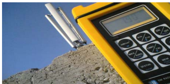
Fig.1 –Picture of the BTS and Equipment, during the measurement
